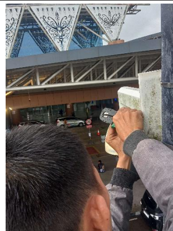
Uraian: Harwat Outdoor PTZ Camera CCTV Objek Vital Keterangan: Maret 2025
